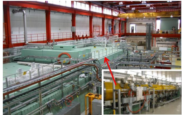
SRF Test Facility is now testing the first U.S. 1.3 GHz cryomodule.
