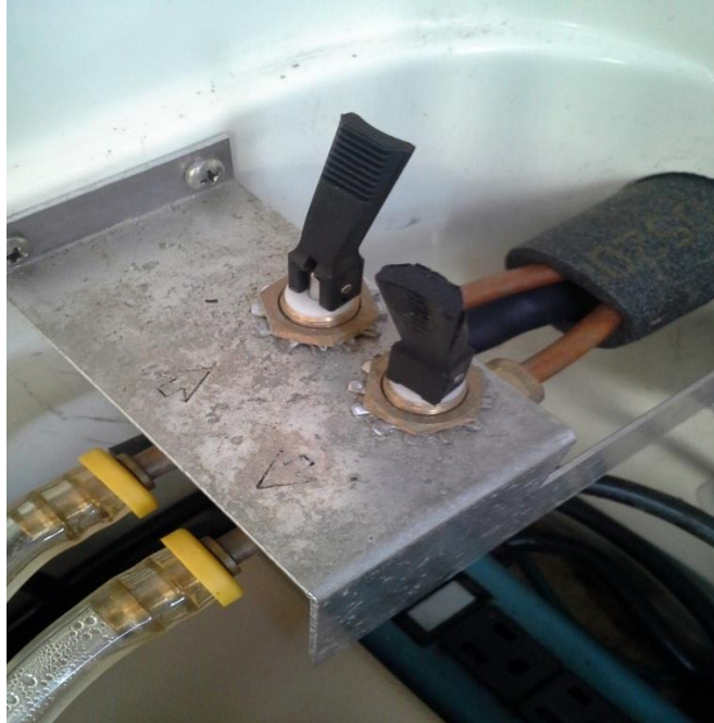
Figure F-3. Picture of the valves connecting the inlet and outlet of the sample tubes to the tritium sampler. When open the handles are in the vertical position.
