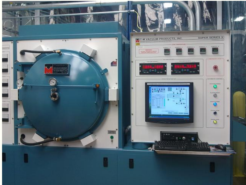
Vacuum furnace in IB4 (Max temp 1000°C)
