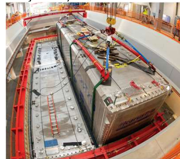
ICARUS physical structure with two cryostats inside a containment chamber, each filled with liquid argon (LAR) and housing detector volume. [1]
