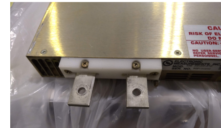
exposed bus on EMS
