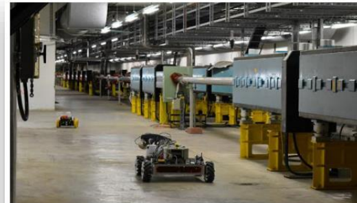
(a) The two robots in the accelerator tunnel navigating to the water leak location seen from the safe human station
