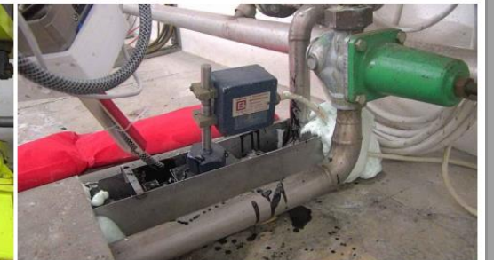
(d) The pouring of the resin in the built metallic box for the water leak fix robot
