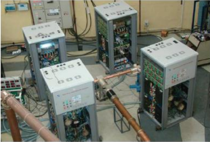
RF station # 3 at 30 kW
