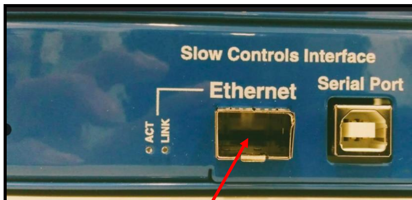
The SFP Slow Control input is bent, preventing the correct insertion of the SFP Module.
