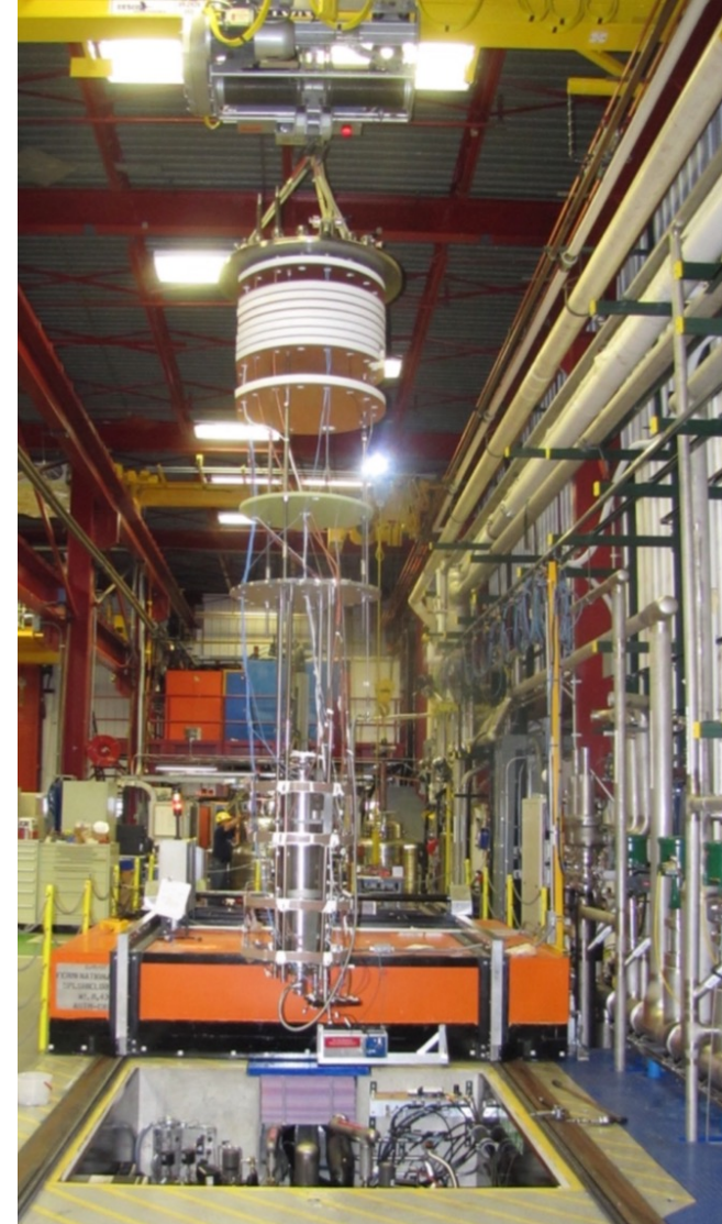
Fermilab Vertical Test Stand used for liquid helium tests of accelerator SRF cavities
