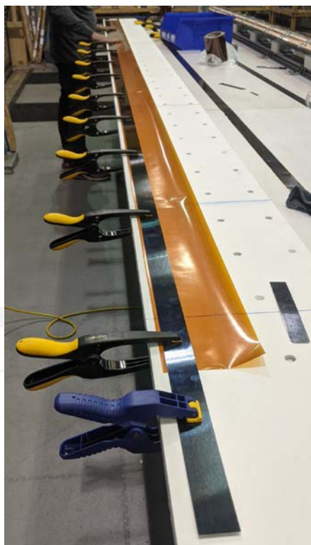
Figure 16: Clamp the metal down on the Kapton. Kapton is epoxy side up.
