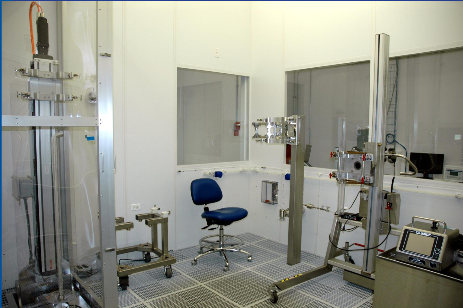
HPR Tool, Clean Assembly Rail, Cavity Carts
