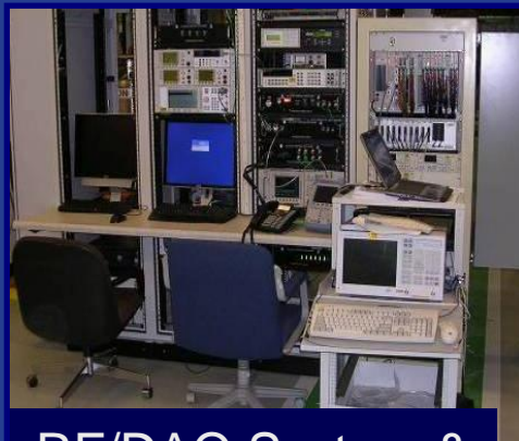
RF/DAQ System & Control Room
