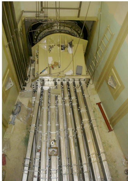
Guide Array in Reactor
