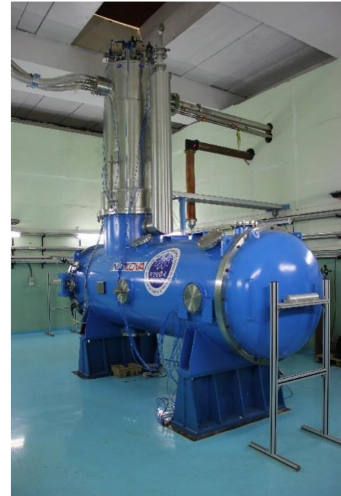
HTS Cryostat Installed at RRCAT
