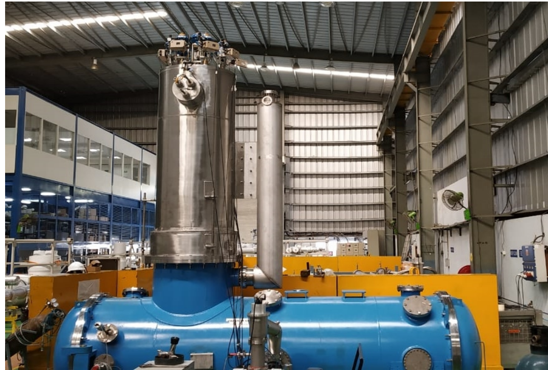
HTS Cryostat at INOXCVA
