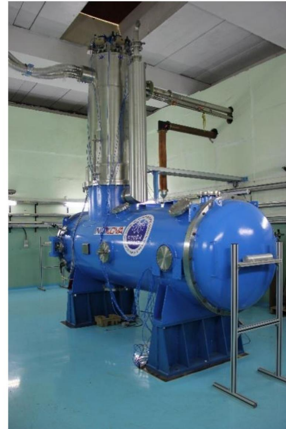
HTS Cryostat Installed at RRCAT
