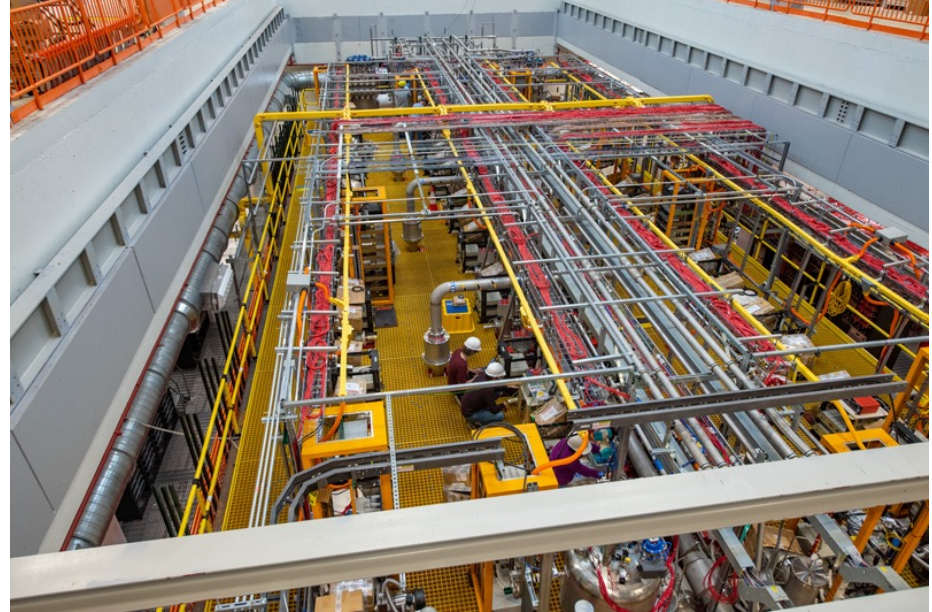
The top of the ICARUS detector before the installation of the Top CRT and overburden systems.
