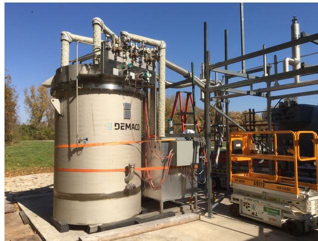
LAr filter in place at SBN ND
