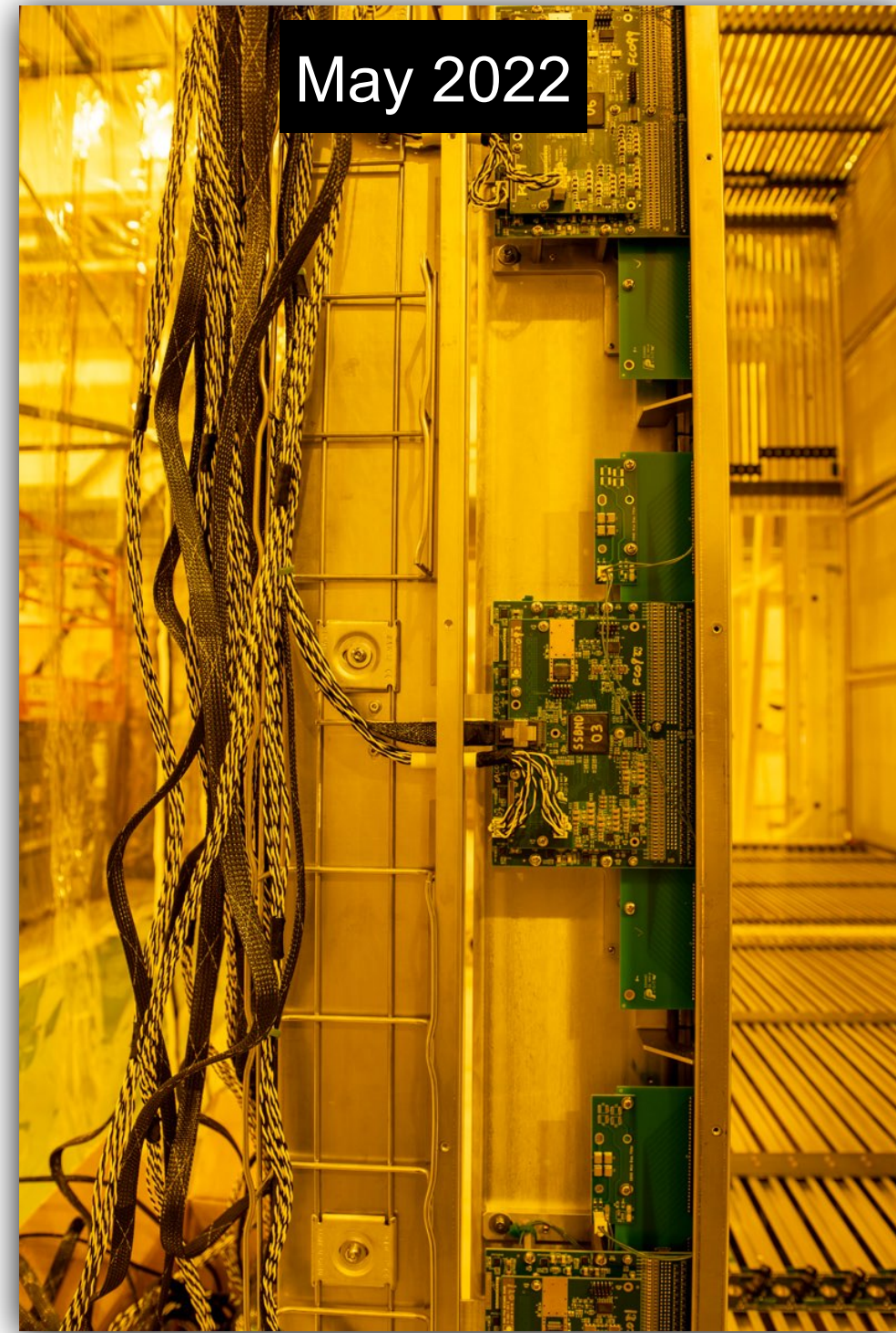
TPC Cold Electronics Installed and tested
