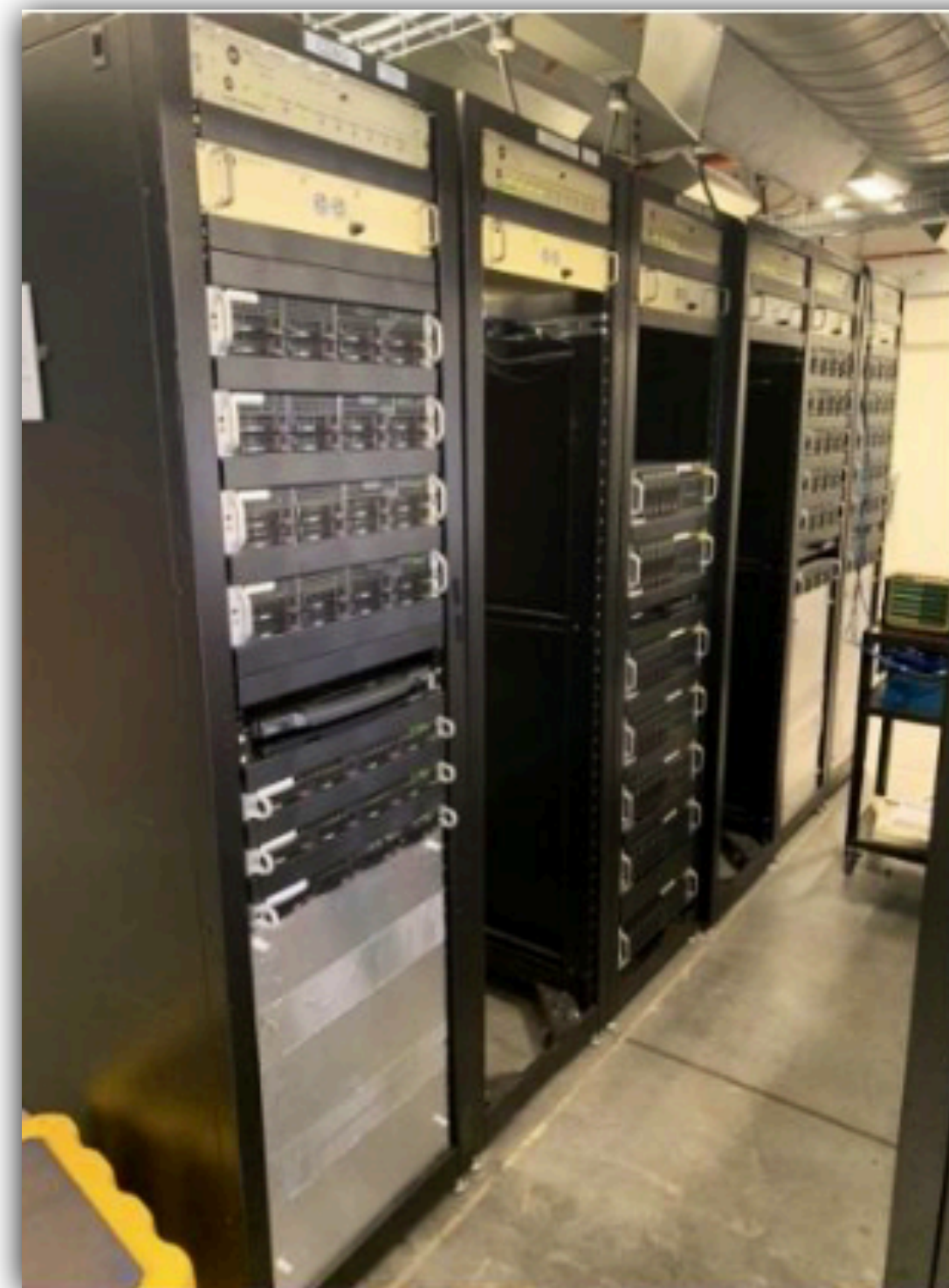
Online server racks
