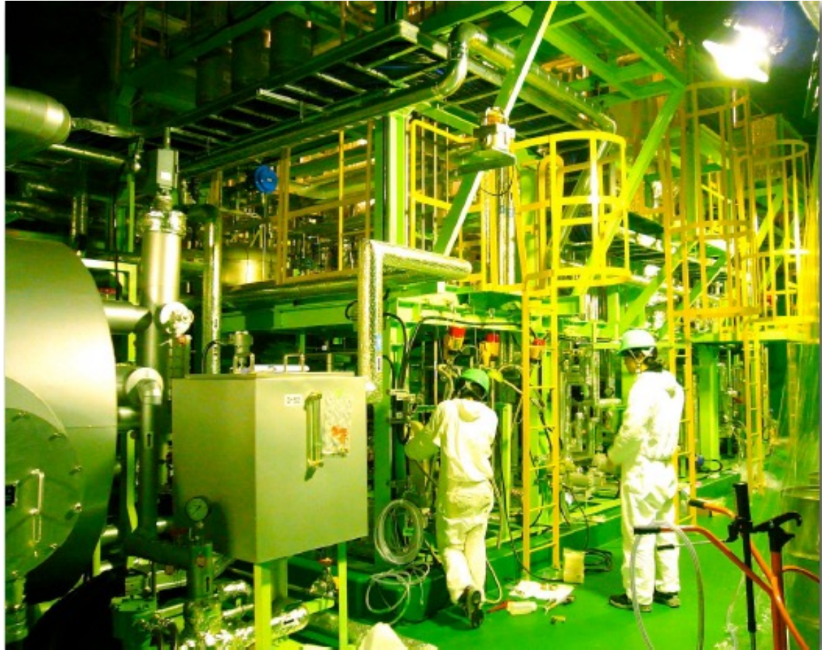
LS and BO purification plant.
