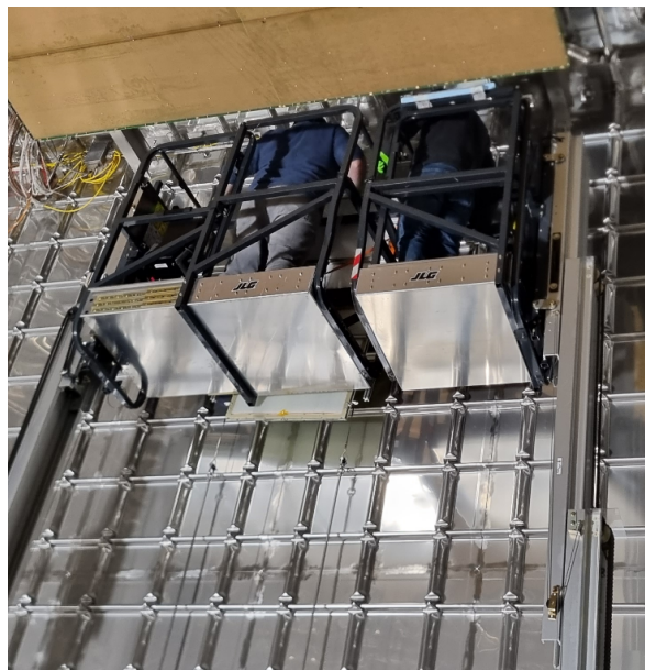
Figure 36. Picture of the two operators at the two scissor lifts during the installation.
