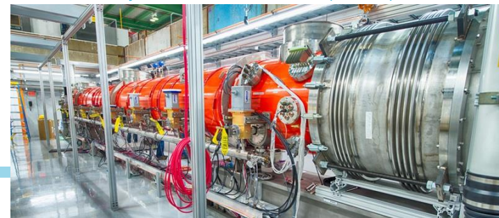
Cryomodule Test Stand (CMTF)
