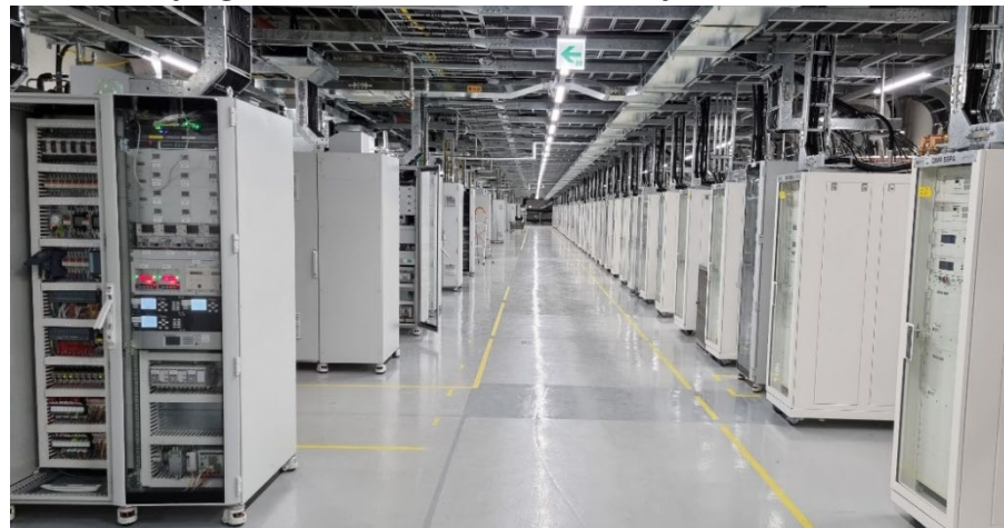
CM/Cryogenic Control Rack and SSPA
