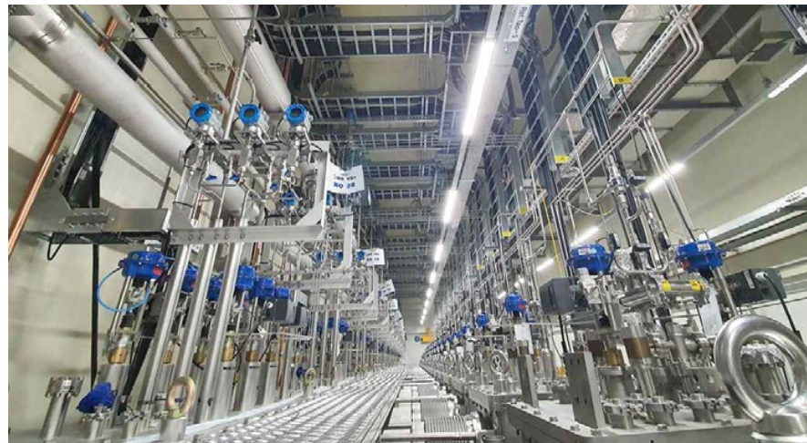
Cryogenic Distribution to Cryomodule
