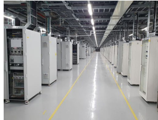
SCL3 Control System(43)
