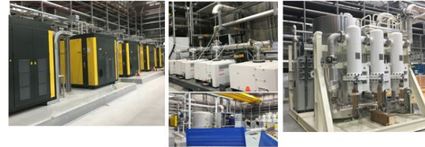
Compressors and Oil Removal System (WCS)
