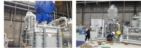
Compressors and Oil Removal System (WCS)
