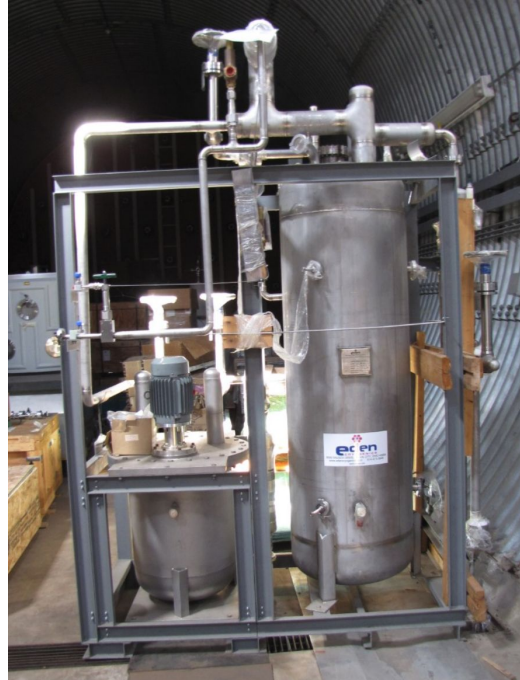
Filter skid (MicroBooNE design): 4A molecular sieve material to remove water contamination and Cu Alumina to remove oxygen contamination. Ten ton LAr recirculation turn over time of ~three hours.
