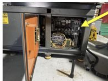
Injection Molding Machine, open control panel showing machine switched off
