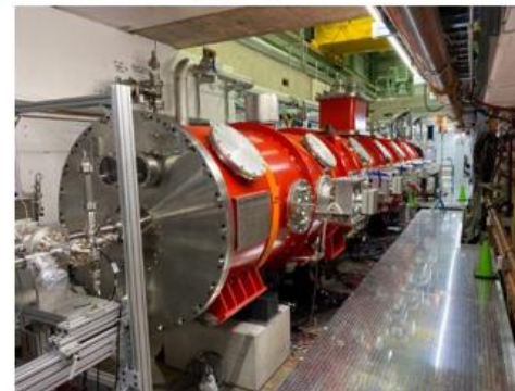
pHB650 Cryomodule installed at 650 Test Stand (Feb. 2023)
