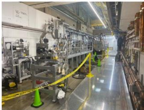
PIP2IT Test Stand infrastructure installed (Nov. 2022)
