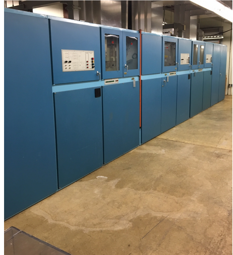
Rectifier inside a service building
