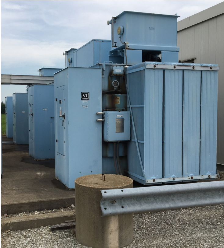
Transformer outside of a service building
