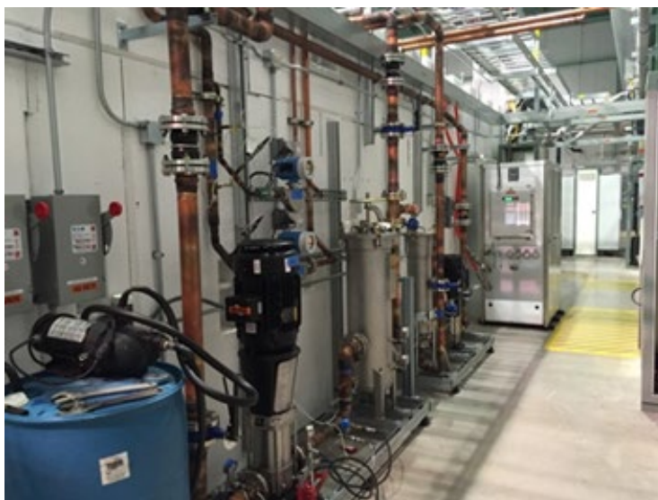
Figure 3-2. RFQ water skids and piping are in the center of the image. The IS chiller system is to the right of the RFQ skids.
