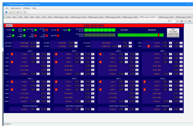
Figure 1-8. An EPICS IOC was tested for SSR1 amplifier control, status, and readback.
