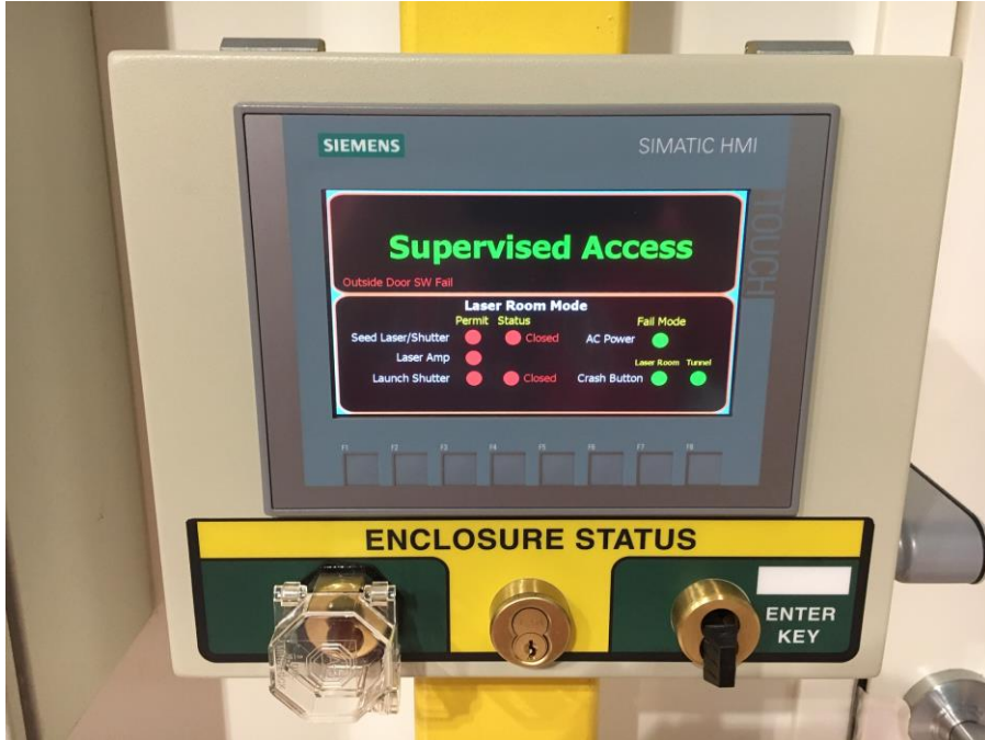
PIP2IT Laser Interlock access control and status
