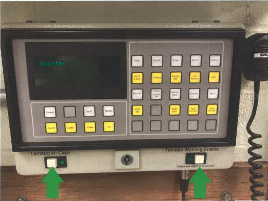
Figure 1: Paging Station – Tornado Warning (see green arrows)
