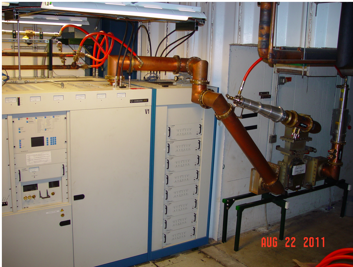
650 MHz Comark 30 kW IOT with Ferrite Circulator @ MDB For Horizontal Test Stand
