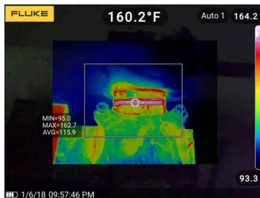
Figure 34: Thermal imaging of the busbars (71,2°C). © Victor Grzelak, Fermilab
