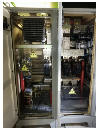
KLOE PS Dump resistor and contactors
