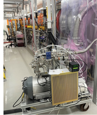
Vacuum cart – connected to Endcap side
