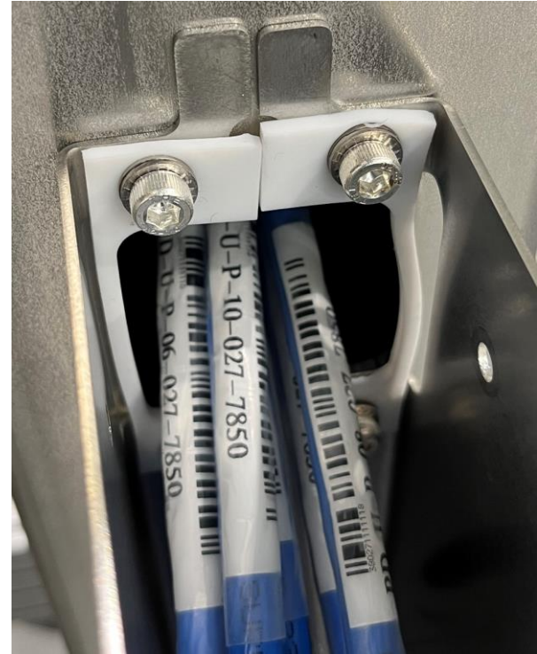
Cables entering APA foot tube Showing grommet deformation
