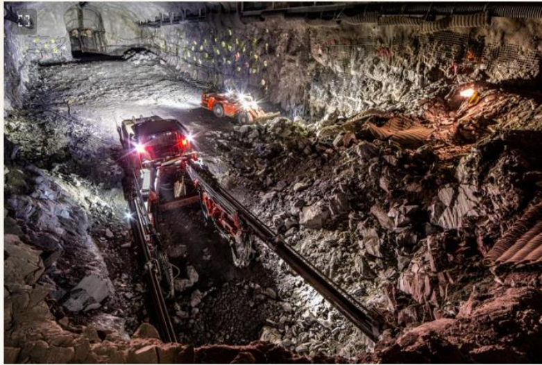
A drill and mucker are seen excavating for the Deep Underground Neutrino Experiment at the 4850 Level at SURF. Photo by Matthew Kapust, Sanford Underground Research Facility
