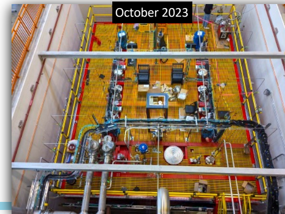
Cabling and cryogenic connections
