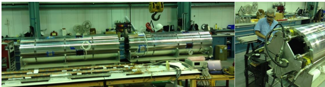
Fig. 4.7. Left: Two half-length yoke-shell subassemblies, ready to be joined. Right: hydraulic rig for pre-tensioning the yoke tie rods.
