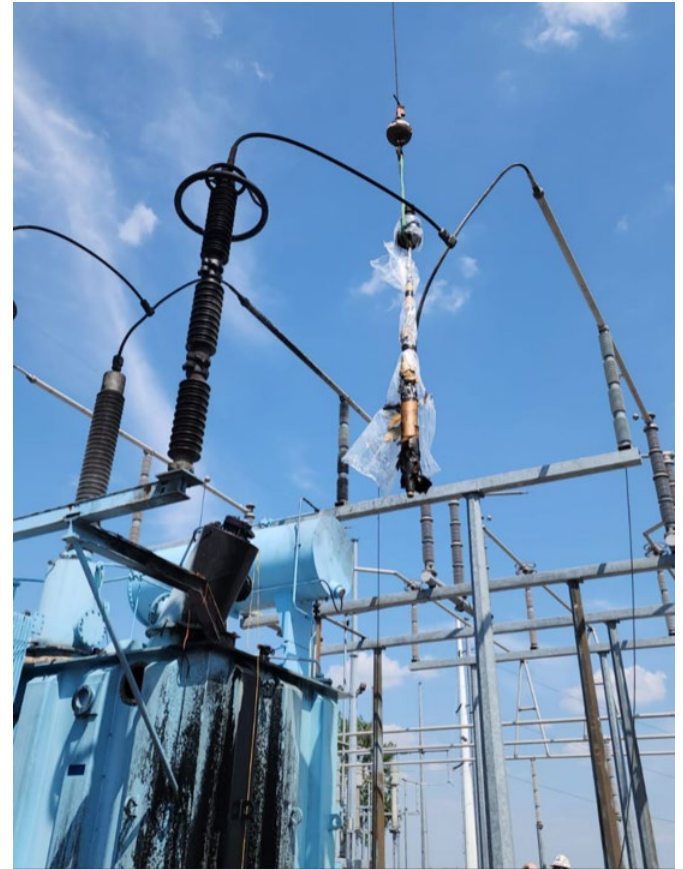
PIC 4 T-88 FAILED BUSHING - PIC 2
