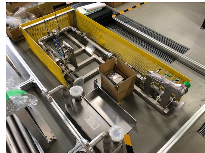
New target cooling system
