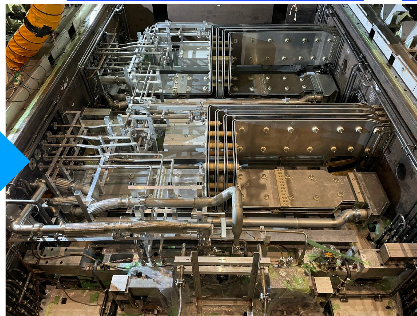
Modified target plumbing
