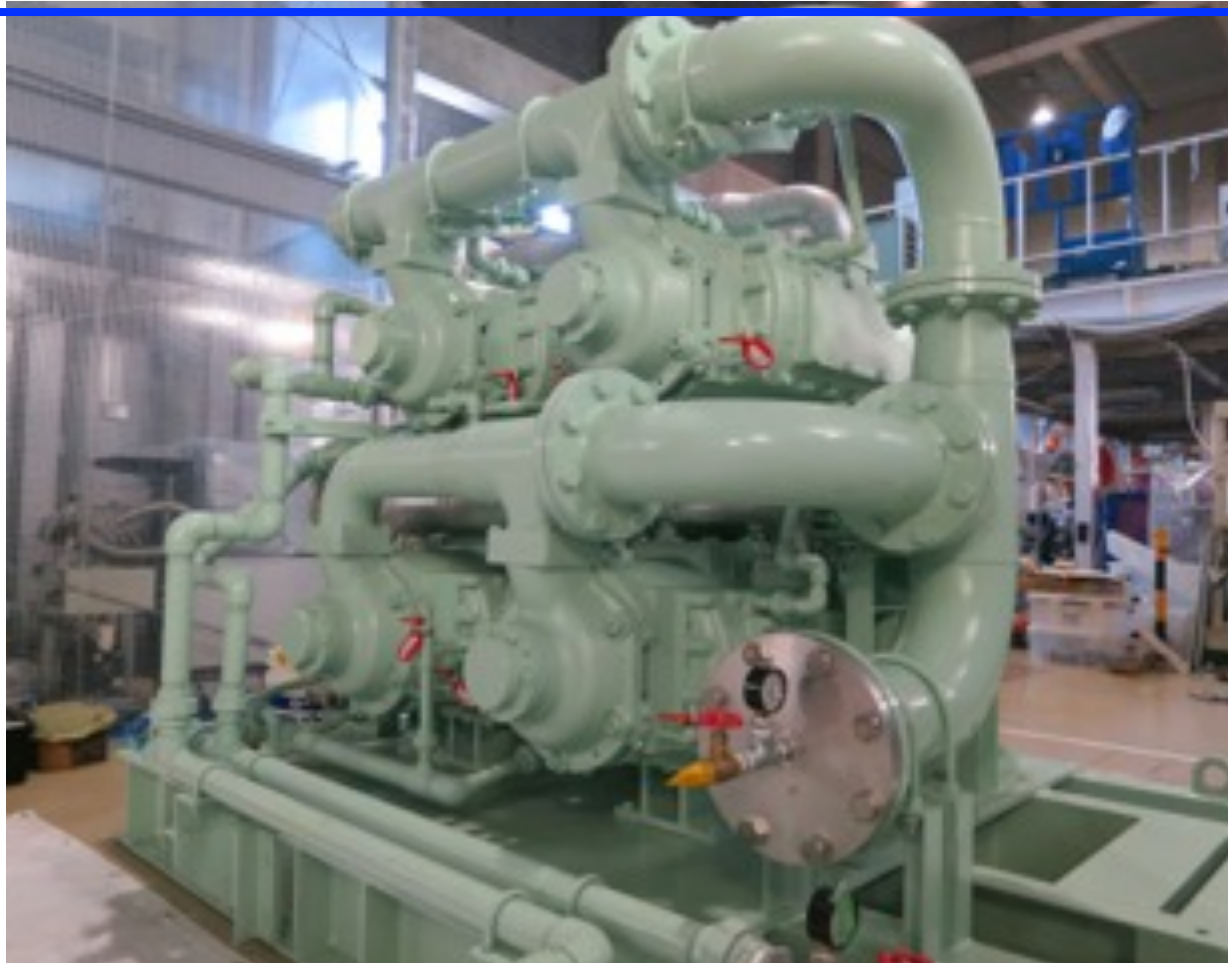
He compressor before installation in 2017
