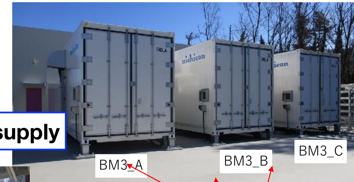
Capacitor Banks for BM3
