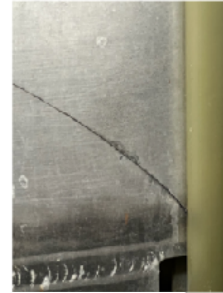
A crack was found on the walkway stripline near Horn 2
