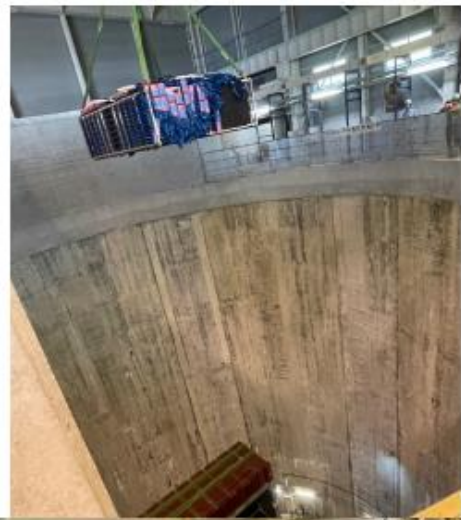
Super-FGD installation (October 2023)
