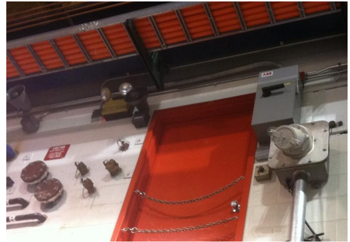
6 th floor counting house utility connections
