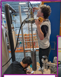
Purity monitoring installation
