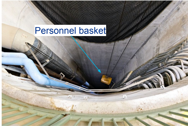
Existing personnel basket in use.
