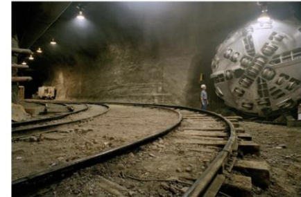
A tunnel of the Superconducting Super Collider project in 1993, which was abandoned by Congress. Ron Hefflin/Associated Press
