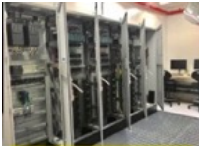
PLC Based Process Controls
