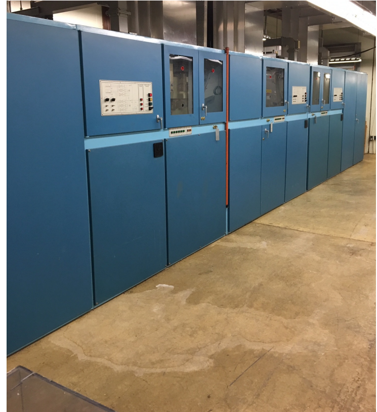
Rectifier inside a service building
