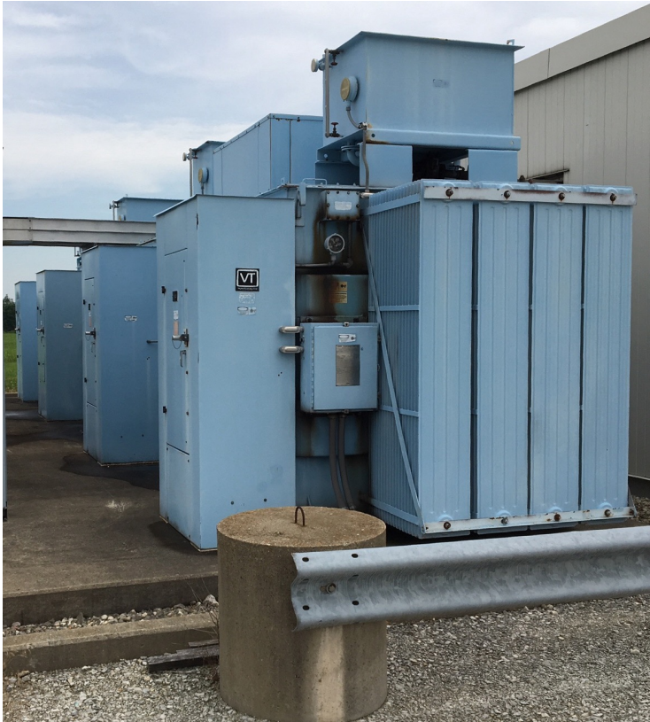
Transformer outside of a service building
