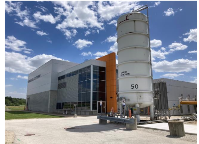
LN2 storage, for cooling.
