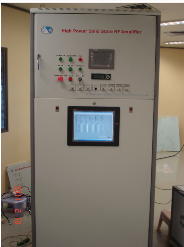
Front View of 8 kW SSPA
