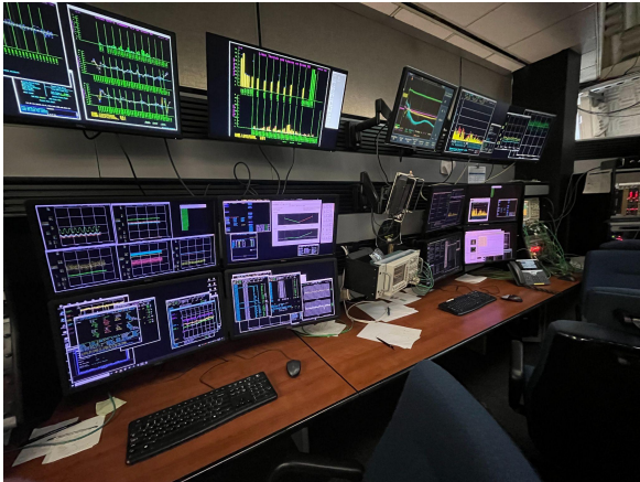
Main Control Room
