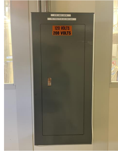
POWER PANEL FACE
